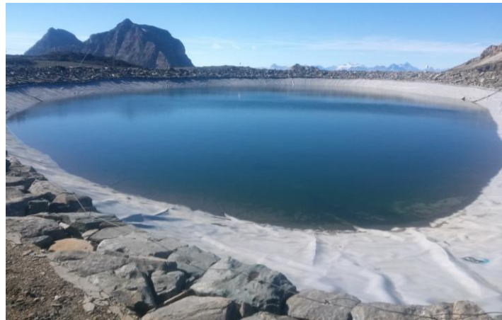
Figure 1 – PVC geomembrane of an altitude reservoir dedicated to the production of artificial snow ; geomembrane showing repairs due to damage by puncturing actions
