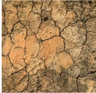
Figure 1: Desiccation cracks in clayey soils.
